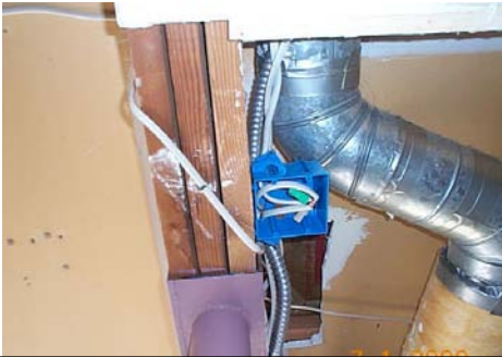
PHOTO #3 HOLE IN SHEETROCK AT GARAGE CEILING/FIRE WALL. MISSING COVER AT JUNCTION BOX
