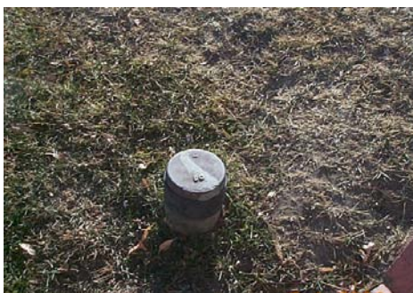
PHOTO #15 WASTE CLEAN OUT EAST
