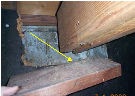
PHOTO #11 GIRDER IS NOT BEARING ON FOOTING AT SOUTH NEAR LIVING ROOM FIRE PLACE.
