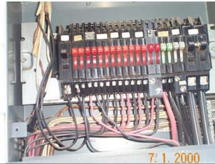
PHOTO #12 ELECTRICAL PANEL SOUTH
