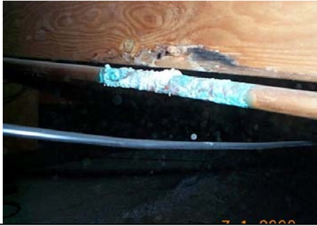
PHOTO #9 LEAK AT SUPPLY LINE UNDER KITCHEN AT CRAWL AREA- NAIL PENETRATED PIPE
