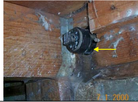
PHOTO#10 LEAK AT CLEAN OUT AREA UNDER KITCHEN SINK AT CRAWL AREA
