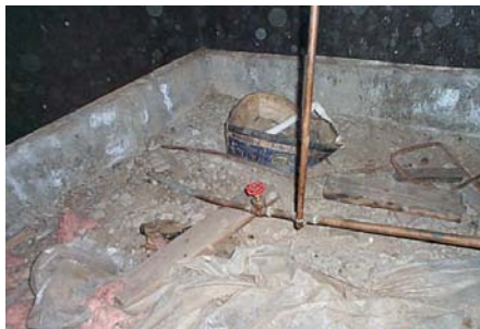
PHOTO #13 WATER SHUT OFF AT CRAWL AREA EAST
