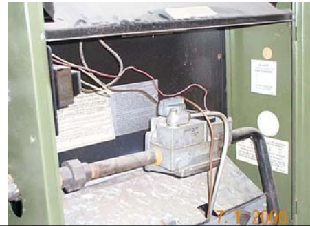
PHOTO #4 HEATER AT GARAGE
