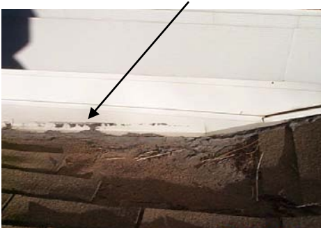
PHOTO #7 MAINTAIN SEALANT AT WALL TO ROOF UNION ABOVE KITCHEN
