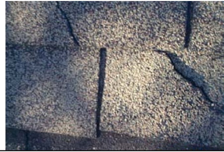
PHOTO #6 CRACKS, BRITTLE SHINGLES AT TOP LAYER AT SOME AREAS
