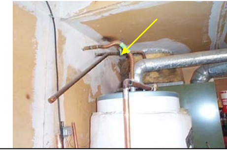
PHOTO #5 LEAK AT WATER HEATER COLD WATER SHUT OFF VALVE
