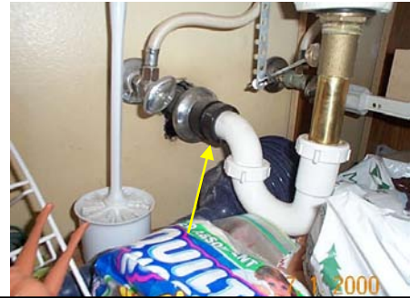
PHOTO#2 LEAK AT TRAP ARM UNDER BATH SINK UP STAIRS
