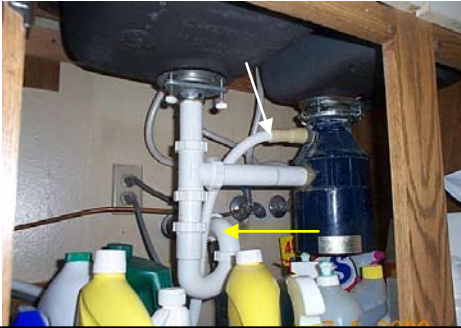
PHOTO #1 LEAK AT TRAP ARM UNDER KITCHEN SINK, NO LOOP OR AIR GAP IN DISHWASHER DRAIN
