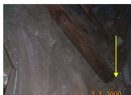
PHOTO #8 EARTH TO WOOD CONTACTS UNDER HOME AT KITCHEN & FOOTING UNDER KIT.
