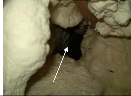
PHOTO#58 OPEN CHASE, NO FIRE DRAFT STOP. NEAR DINING ROOM/ENTRY
