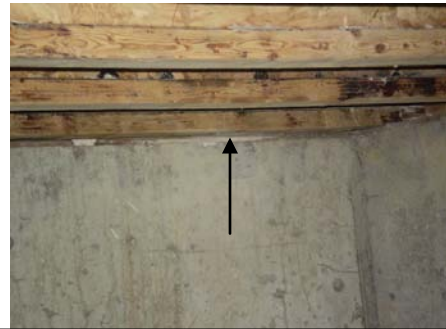
PHOTO #60 SOME FOUNDATION VENTS ARE BLOCKED BY JOISTS AT INTERIOR- NO INSULATION
