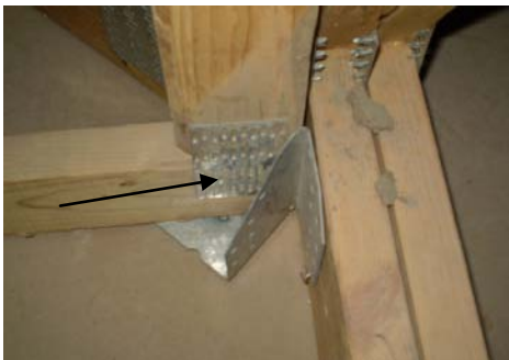
PHOTO #55 IMPROPER HARDWARE AT SOUTH ABOVE GARAGE. NO NAILS OR FASTENERS
