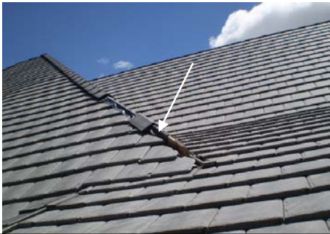
PHOTO #51 MISSING, DAMAGED TILE. INCORRECT WEATHER BLOCKING
