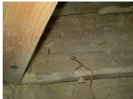
PHOTO #4 ABANDONED WIRES IN ATTIC- NEAR NOOK
