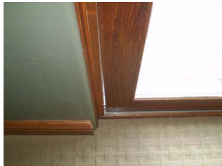
PHOTO#26 DOOR FRAME IS OUT OF SQUARE AT FAMILY ROOM
