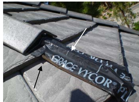
PHOTO #48 MISSING NAILER AT HIP. GAPS AT WEATHER BLOCKING WHERE WATER ENTERS
