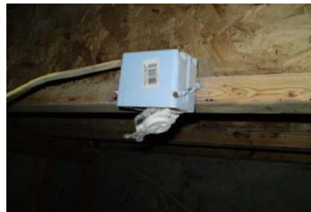
PHOTO #6 LOOSE OUTLET, INCOMPLETE WIRING, MISSING COVER UNDER ENTRY
