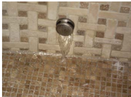
PHOTO #12 WATER FLOWS FROM MR. STEAM, NOT STEAM
