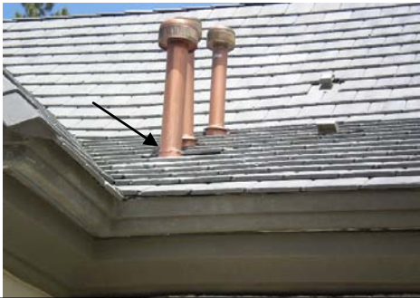
PHOTO #43 MISSING STORM COLLAR, LIFTED TILES, SOUTH
