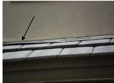
PHOTO #44 LIFTED WALL TO ROOF FLASHING
