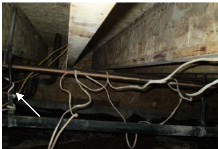
PHOTO #5 UNSUPPORTED WIRES, ABANDONED WIRES- CRAWL AREA BELOW KITCHEN
