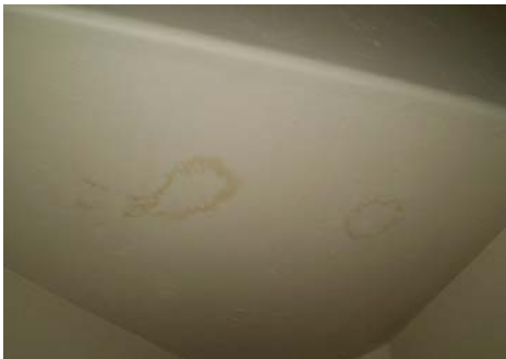
PHOTO #25 WATER DAMAGE AT MASTER BEDROOM CEILING FROM ROOF LEAK ABOVE
