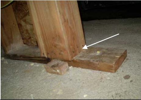
PHOTO #65 PLANS SHOW 6x10 POST, POST IS 6x6- NO POST BASE BRACKET. COMPRESSION AT SILL
