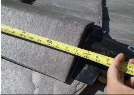
PHOTO #49 15" EXPOSURE ON SOME TILES
