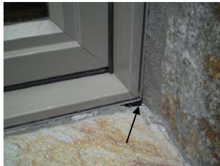
PHOTO#34 SEALANT NEEDED AT WINDOWS AND DOORS TO PREVENT WATER ENTRY
