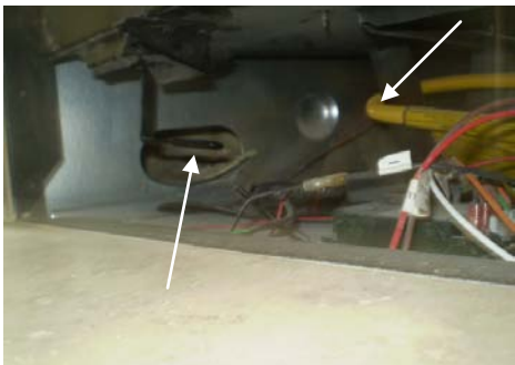
PHOTO #11 FLEX GAS LINE RUGS ON SUPPORT AT MASTER FIREPLACE. FOAM INSULATION BLOCKS AIR FLOW
