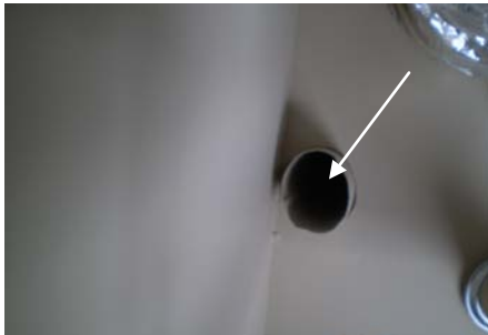
PHOTO #21 HOLE INTO ATTIC ABOVE WATER HEATER. NO FIRE DAMPER. HOLE IN FIRE WALL
