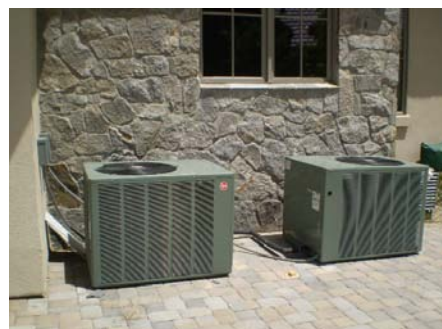
PHOTO #8 AC UNITS SOUTH
