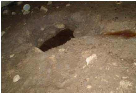
PHOTO #61 STANDING WATER, MUDDY SOILS.
