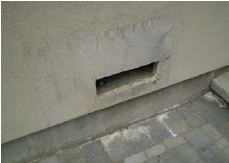
PHOTO #59 FOUNDATION VENTS ARE MISSING AT 2 LOCATIONS EAST
