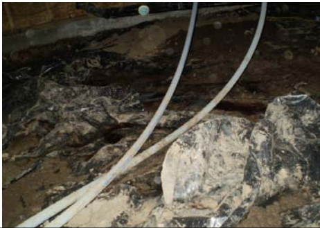
PHOTO #19 UNSUPPORTED WATER LINES.
