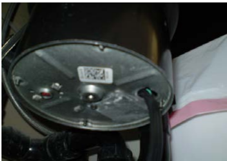
PHOTO #3 WIRES NOT SECURED TO DISPOSAL AT KITCHEN SINKS- (2)
