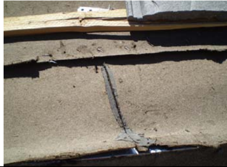
PHOTO#50 ORIGINAL DAMAGE TO FELT WAS PATCHED INCORRECTLY.
