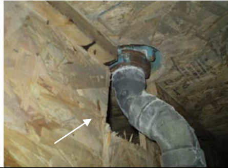
PHOTO#66 CUT FLOOR JOIST UNDER WEST BATH SHOWER
