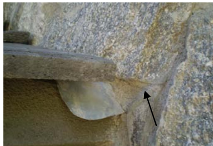
PHOTO #30 DIVERTER IS BURIED IN STONE AND MORTAR- WEST
