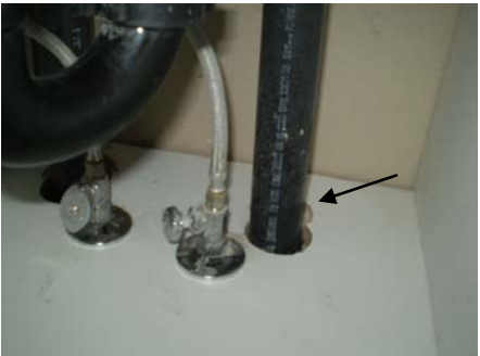
PHOTO #24 HOLES IN CABINET BASE. AIR FLOWS FROM CRAWL AREA. NO INSULATION
