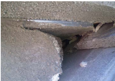
PHOTO #27 HOLE IN EAVE. BIRD, ANIMAL ACCESS TO ATTIC
