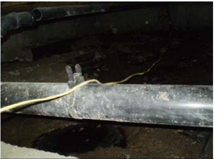
PHOTO #20 BROKEN PLUMBING SUPPORT, CENTER. LOOSE WIRES, STANDING WATER
