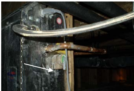
PHOTO #13 NO DRAIN LINE ON MR. STEAM TO VALVE IN CRAWL AREA
