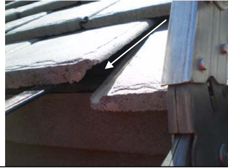
PHOTO#42 RANDOM CHECK OF EDGE TILE. MISSING WIND CLIPS
