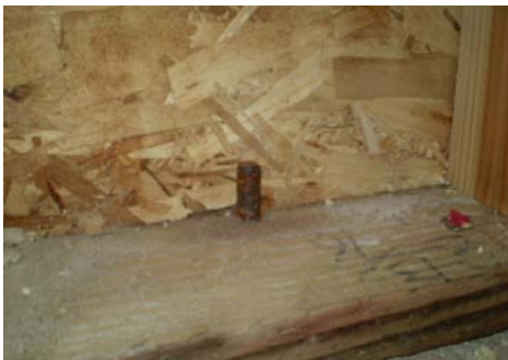
PHOTO #63 MISSING NUT/WASHER AT ANCHOR BOLT BY POST SHOWN IN PHOTO #64
