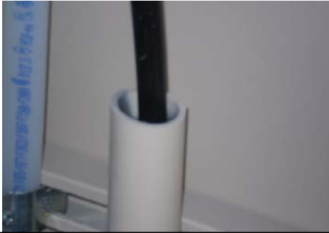
PHOTO #17 WATER SOFTENER DRAINS DIRECTLY TO WASTE LINE. NO ANTI-SIPHON OR BACK FLOW DEVICE VISIBLE- GARAGE
