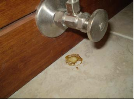
PHOTO#18 LEAK AT SOUTH BATH TOILET SUPPLY LINE
