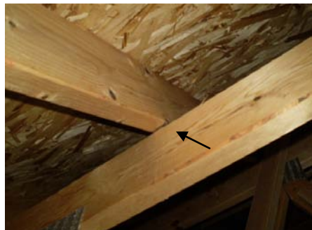
PHOTO #56 NO HARDWARE, NAILS OR CONNECTORS AT HIP TRUSS TO RAFTER ABOVE
