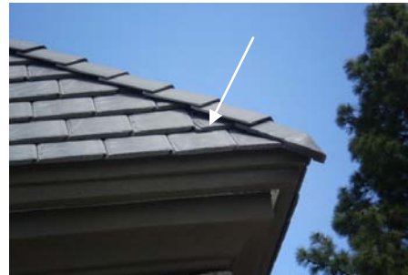
PHOTO #46 SHIFTED TILE. LOOSE TILE
