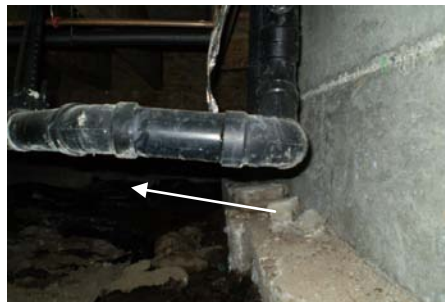
PHOTO #14 WASTE LINE FLOWS UP HILL TO EXIT UNDER KITCHEN
