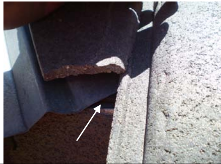
PHOTO #52 VALLEY DOES NOT PROJECT 1" BEYOND ROOF EDGE. BROKEN TILE
