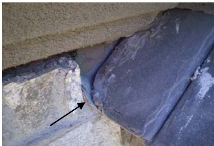
PHOTO #29 DIVERTER DOES NOT PROJECT BEYOND FACE OF STONE VENEER- WEST
