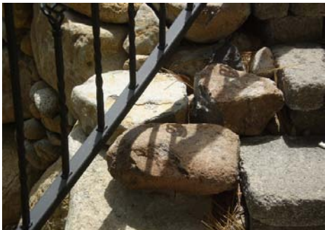
PHOTO #33 HAND RAIL IS NOT ADJACENT TO STAIRS AT NORTH EAST CORNER
