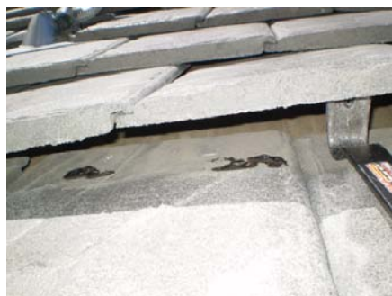
PHOTO #40 RANDOM FIELD TILE HAS NO NAILS INSTALLED. ADHESIVE ONLY
