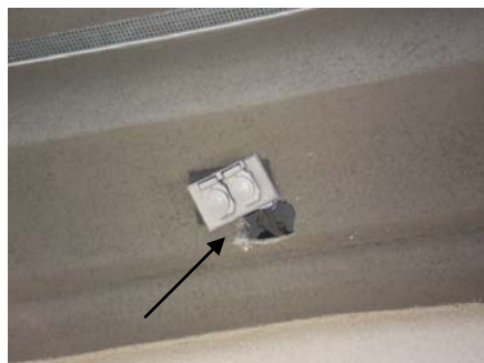
PHOTO #36 HOLES IN SOFFIT AT SEVERAL LOCATIONS
