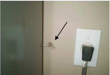
PHOTO #22 NO FIRE CAULKING AT HOLE BEHIND HEATERS AT GARAGE
