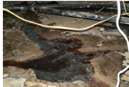
PHOTO #62 STANDING WATER, UNSUPPORTED WIRES.
