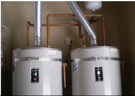
PHOTO #9 WATER HEATERS AT GARAGE. NO DRIP LEGS IN GAS LINES PRIOR TO REGULATORS
