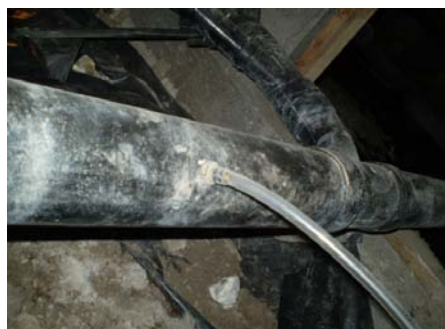
PHOTO #16 FLEX DRAIN LINE TAPS INTO WASTE LINE. POSSIBLE CROSS CONNECTION-
