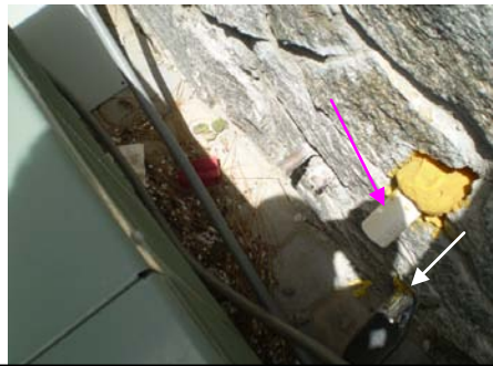
PHOTO#10 NO ELBOWS ON WATER HEATER TP VALVES BEHIND AC SOUTH. NO PAINT AT PVC
