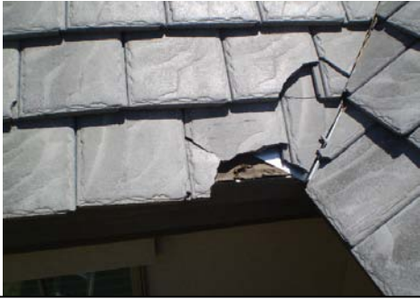
PHOTO #41 FELT DOES NOT PROJECT OVER ROOF EDGE. BROKEN TILE
