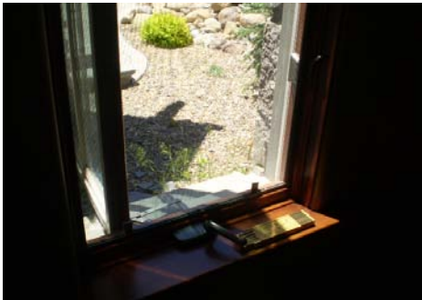
PHOTO #23 WINDOW AT WEST BEDROOM DOES NOT OPEN TO PROVIDE 20" WIDTH FOR EGRESS
