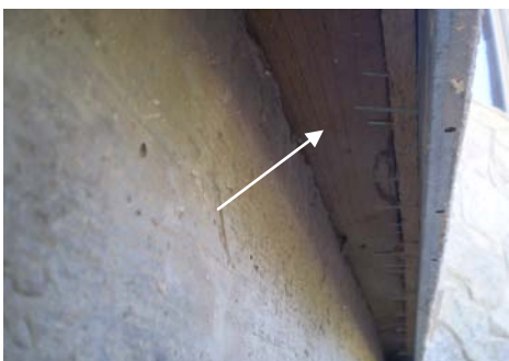
PHOTO #39 MUD SILL IS CANTILEVERED OVER STEM WALL AT WEST
