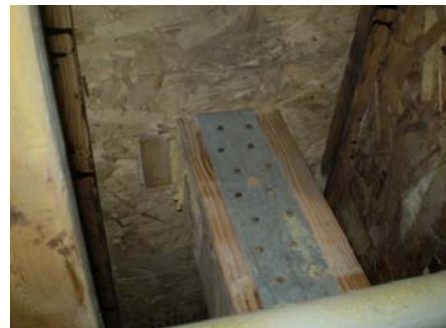
PHOTO #64 6x6 POST IS STRAPPED AT SPLICE. PLANS SHOW 6x10 POST AT THIS LOCATION. NO PB
