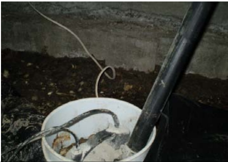
PHOTO #67 INCOMPLETE INSTALLATION OF SUMPS. NO BACK FLOW DEVICE IN WASTE LINE
