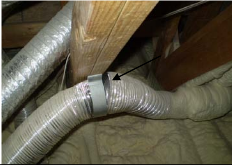
PHOTO #57 DAMAGED EXHAUST DUCT SOUTH
